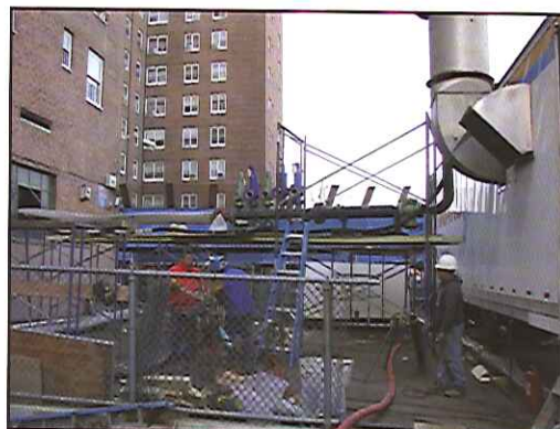
Installation at Red Hook East
