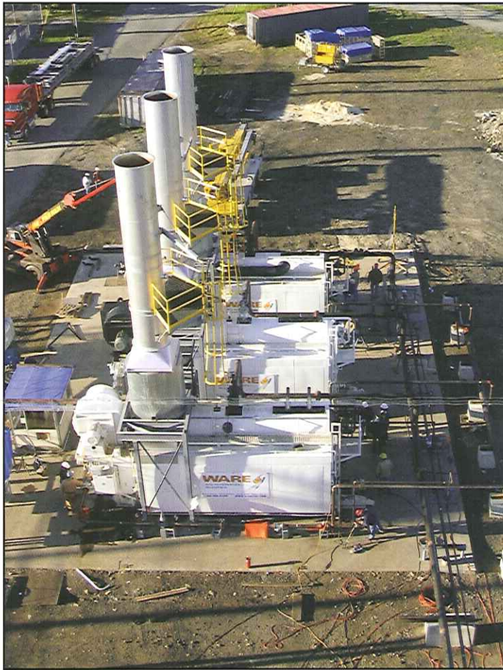
Today's Rental Boilers
